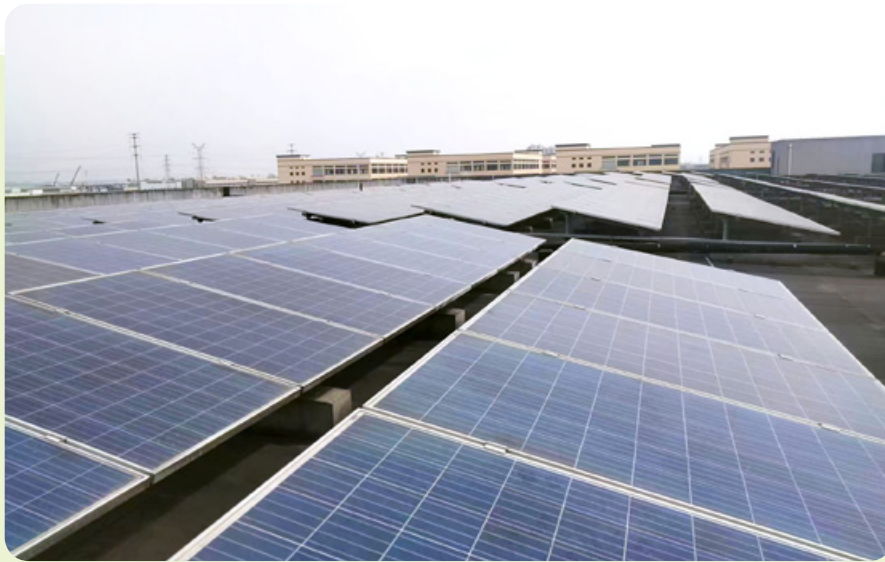
● Photovoltaic power generation facilities of Joyoung
